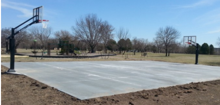
A new concrete basketball court with two adjustable goal posts, has been completed in the Pioneer Day Use Area
